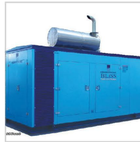
Standby Generator Common area & Lift
